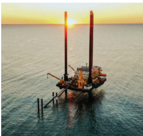
WIND, WATER Vineyard Wind technology will protect marine life (top), while South Fork has new jack-up vessel.
